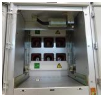
活门打开 Valve open
